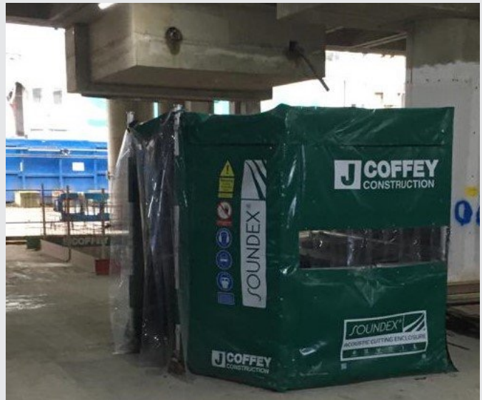
Noise enclosure / barriers used to mitigate noise exposure to other site users
