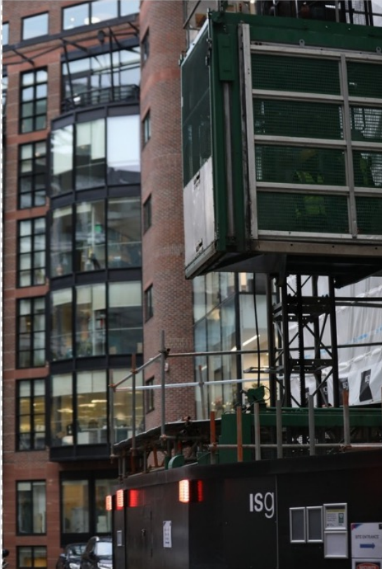
Passenger enclosed type hoist with base segregation
