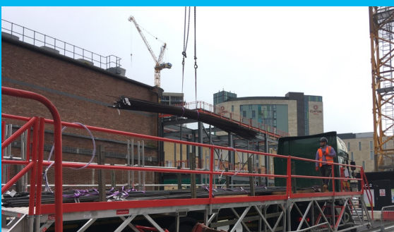
Vehicle unloading handrail system to eliminate work at height
