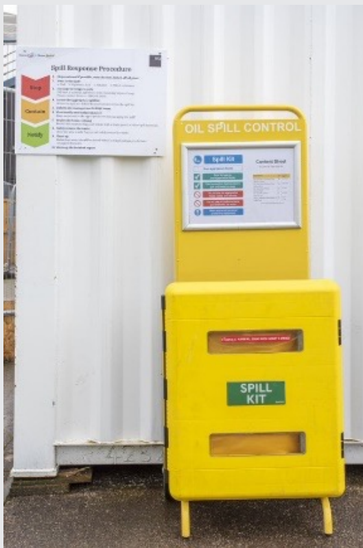
Examples of spill response stations with instructions clearly displayed
